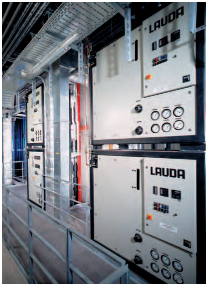
Modular construction of temperature control systems – here in the production center at Nycomed, Singen, Germany
